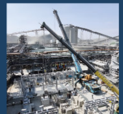
Cover Photo Lycopodium Modular Plant
